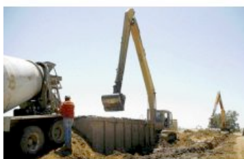
Photos by Nick Adams/Appeal-Democrat Excavators work on the slurry wall being built to reinforce the Feather River levee on the Yuba County side on Thursday. It is part of the final phase of $400 million in levee improvements over the past four years.
